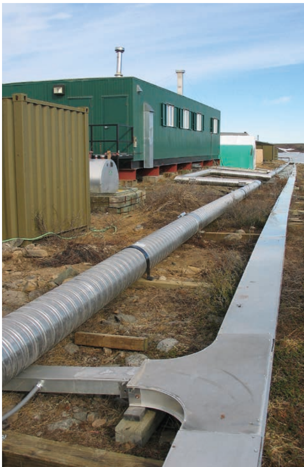
Facility planning can minimise the need for tubing and hence reduce heatloss and energy consumption (Elmer Topp-Jørgensen/Aarhus University).
