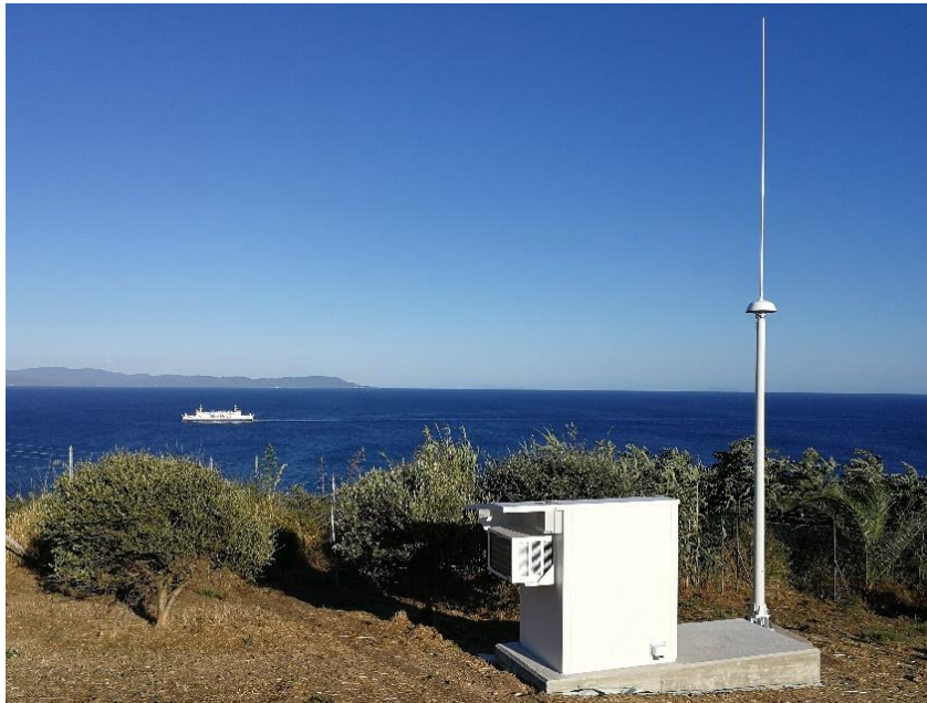
Figure 6-2: compact shelter for HFR station of LaMMA Consortium in Piombino (Italy). Source: SICOMAR Plus project T2.1.2 “production of new datasets from HFR networks”.
