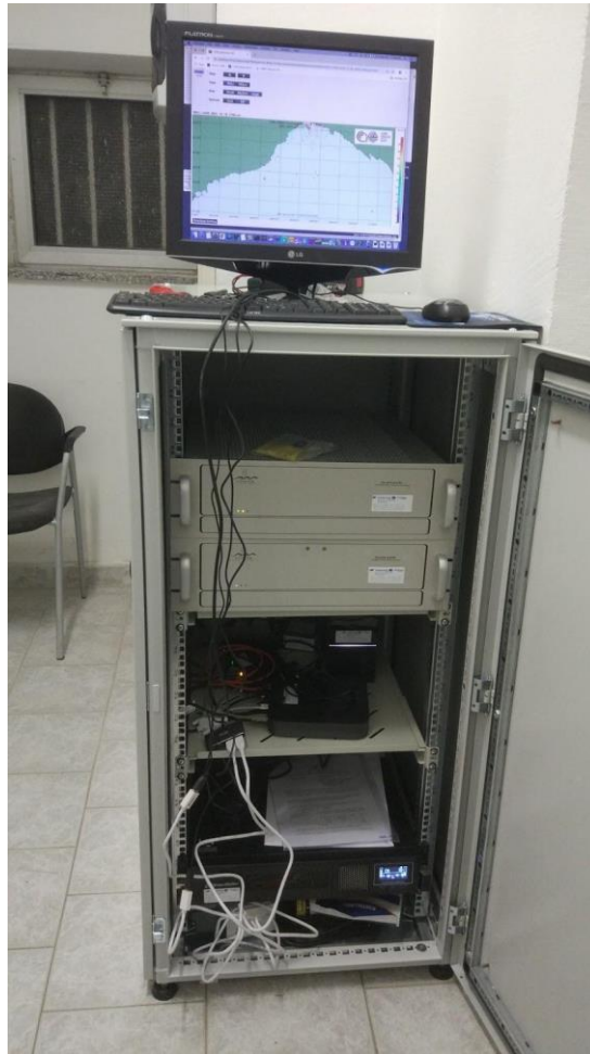
Figure 6-1: Example of rack cabinet hosting HFR units, computers and other accessories. Source: CNR HFR station in Liguria, Italy.
