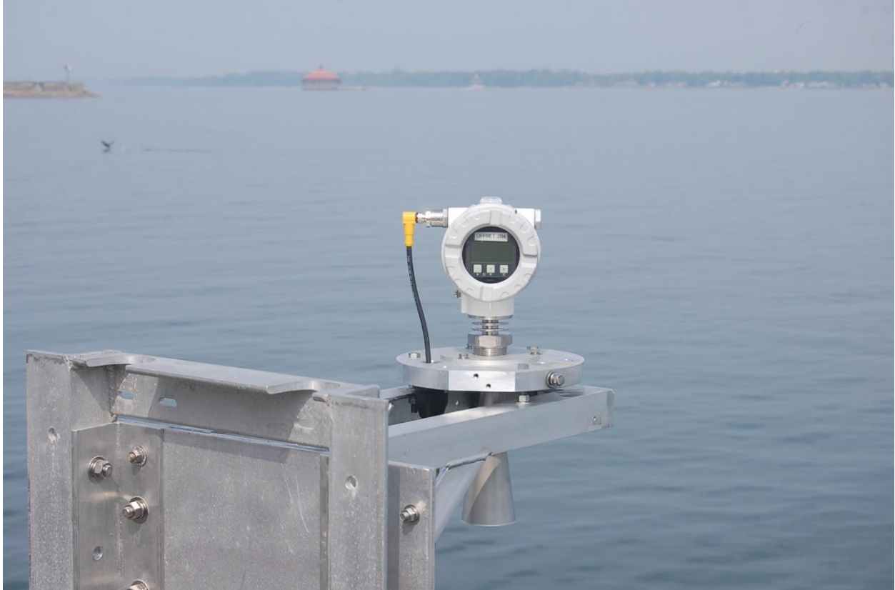
Figure 2-1. Xylem/Design Analysis H3611 microwave water level sensor as installed by NOS/CO-OPS.
