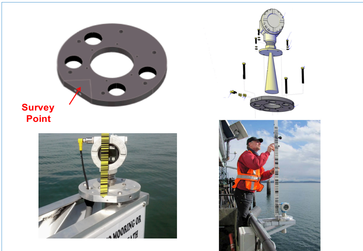
Figure 4.4 The mounting collar used by NOAA for horn radar gauges such as the Waterlog H-3611. The collar is a 1-inch thick disk of aluminium with holes for attachment of the sensor to the collar and of the collar to the supporting frame. A levelling rod can be placed on an area on the top face of the collar to enable geodetic connection to neighbouring benchmarks. (Photographs NOAA).
