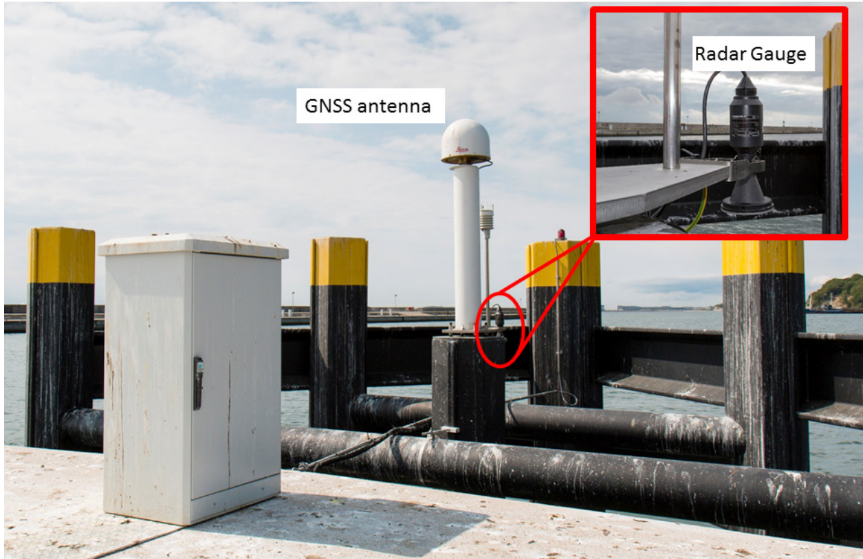
Figure 12 New GNSS reference station in Sassnitz (GREF station SAS2) with GNSS antenna on top of the antenna pillar, control unit, weather measurement unit and Radar Gauge (in operation since April 2016).
