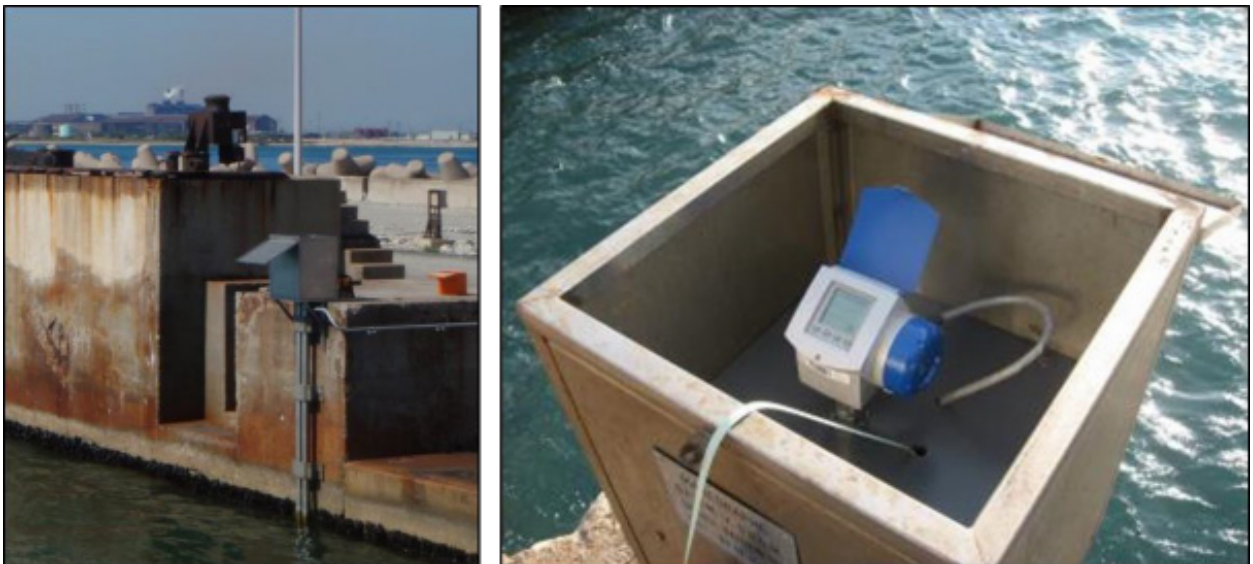
Figure 4. Example of RONIM tide gauge installation. Optiwave mounted in stainless steel stilling well at Fos-sur-Mer (right).
