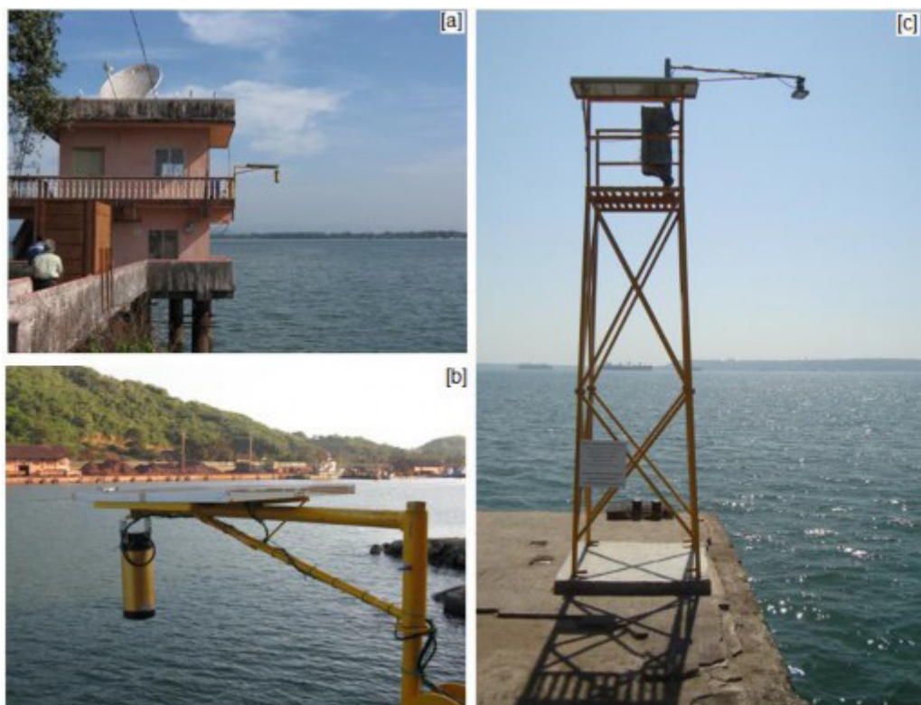
Figure 3. Typical installations of microwave based radar gauges at [a] Karwar, [b] Port Blair and [c] Dona Paula.
