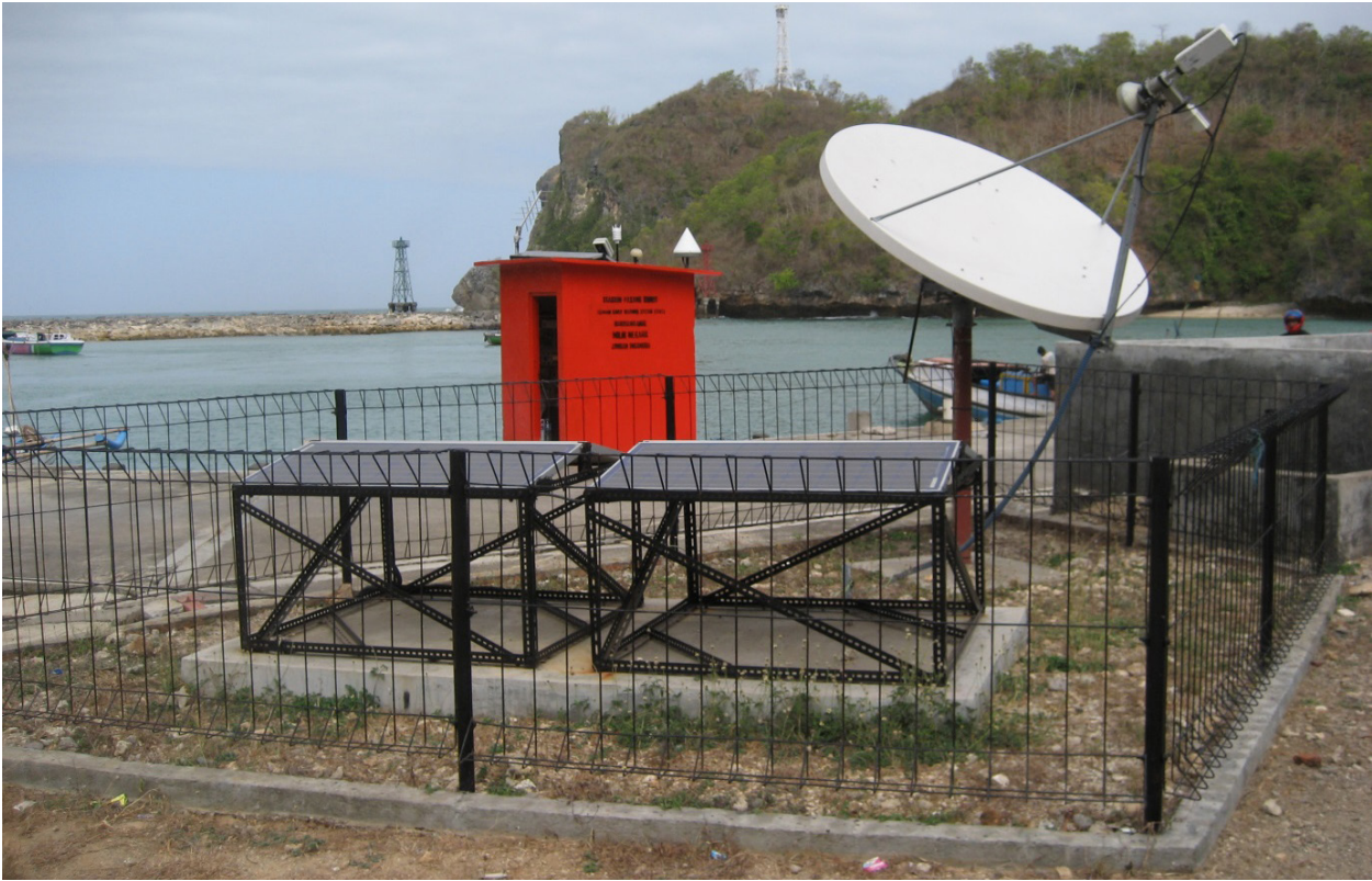
Figure 7.5 A VSAT dish alongside a tide gauge in Indonesia. This station is also equipped with an OTT Kalesto radar gauge and GPS receiver. (Photograph Tilo Schöne, GFZ).
