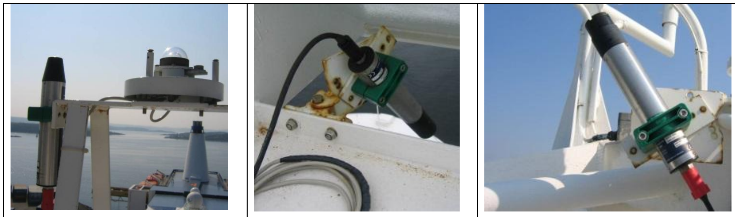
Figure 4.8.1. Installation on a ship of opportunity in Skagerrak. Radiance sensors can be mounted at different place on the ship.
