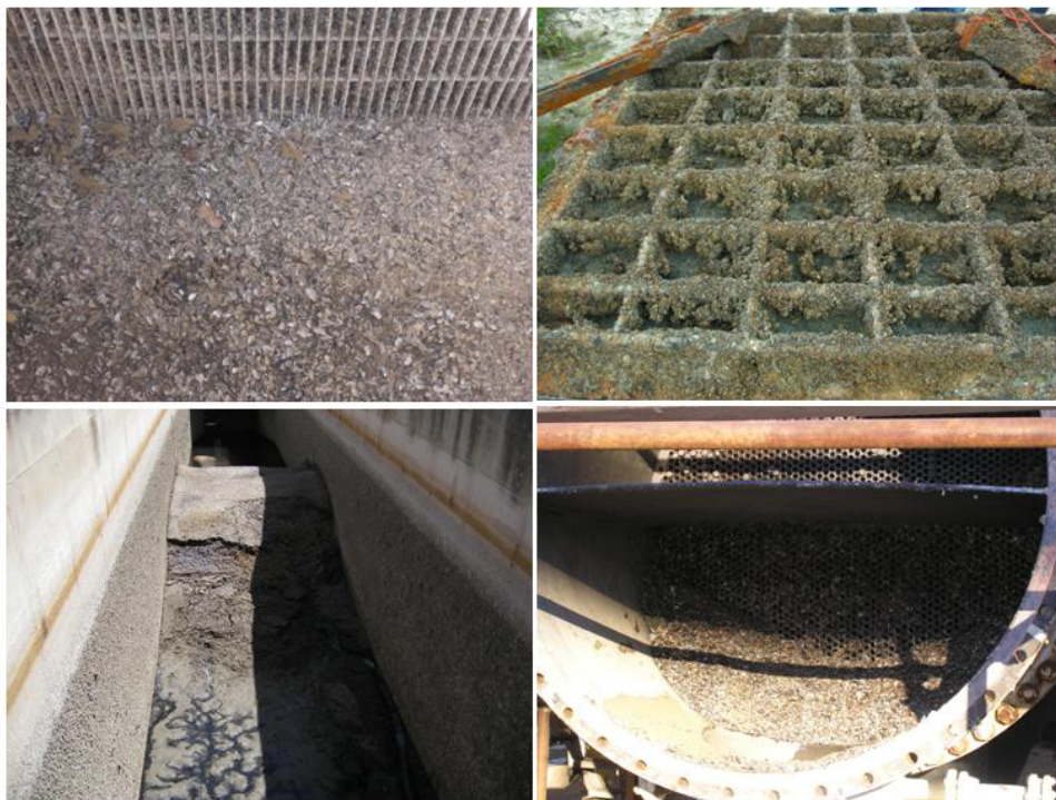
Figure 3.2: Biofouling colonization residual inside cooling water system [1].
