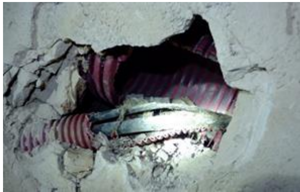
Figure 21. Destruction of optical fiber eaten by rats.
