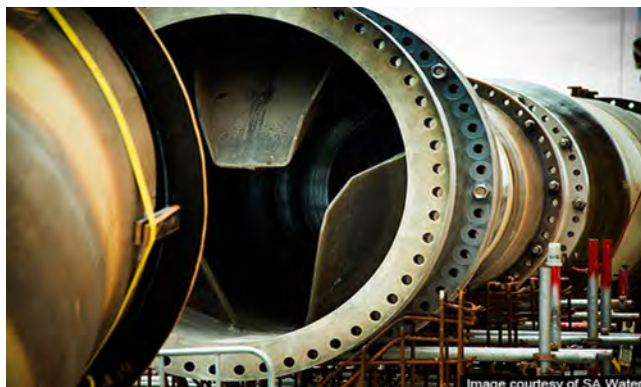
Figure 9.4. In-line static mixer at the Adelaide SWRO desalination plant prior to UF pretreatment. Approximate flow through this mixer is 6,250 m 3 /h.
