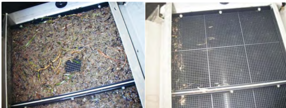
Figure 6.2. Algae and other marine debris blocking the Traveling Water Screens (left) at a SWRO desalination plant in the Indian Ocean and the screens following cleaning (right). Photos: Domingo Zarzo Martinez, Valoriza Agua S.L.
