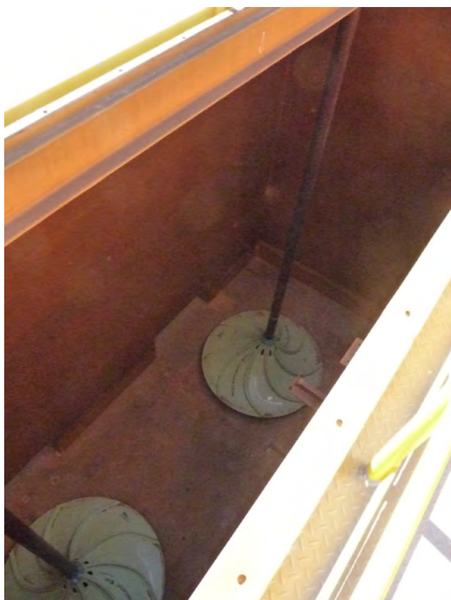
Figure 9.5. Flash mixers in a coagulation tank.
