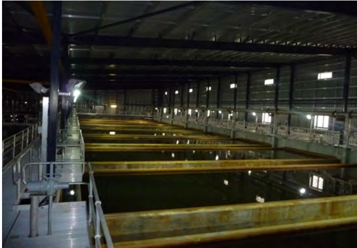
Figure 9.21. Single-stage dual media gravity filters at the Gold Coast SWRO Desalination Plant
