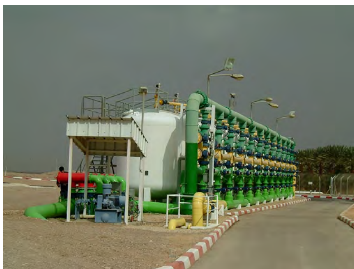
Figure 9.22. Vertical pressure pretreatment filters capacity. Photo: Voutchkov 2013.
