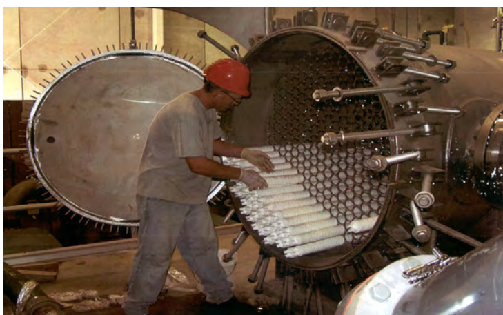
Figure 9.30. Cartridge filters installed in horizontal vessel.
