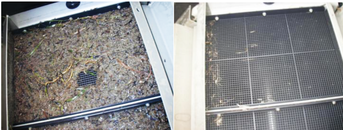
Figure 6.2. Algae and other marine debris blocking the Traveling Water Screens (left) at a SWRO desalination plant in the Indian Ocean and the screens following cleaning (right). Photos: Domingo Zarzo Martinez, Valoriza Agua S.L.
