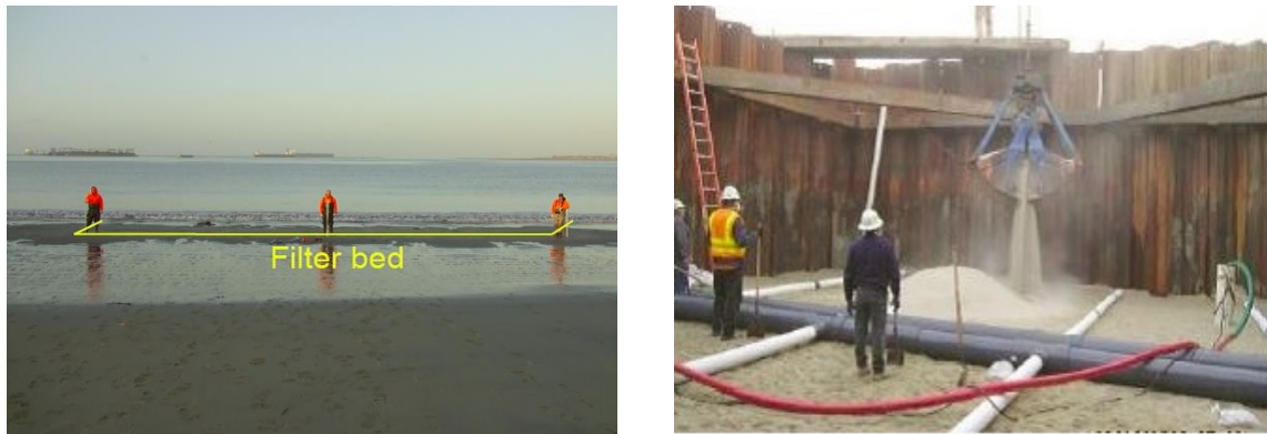
Figure 6.23. Filtration area of under-ocean floor seawater intake (left hand side) and filling of infiltration gallery with engineered sand during construction using a temporary cofferdam (right hand side) at Long Beach (Zhang et al. 2011). Reprinted with permission from American Water Works Association.
