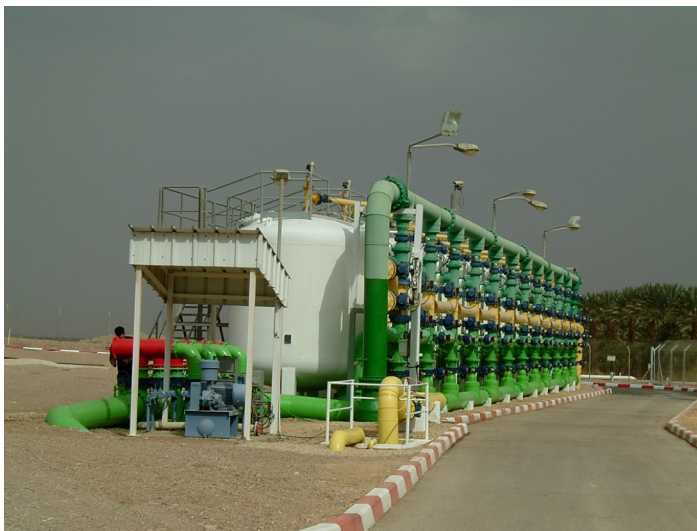
Figure 9.22. Vertical pressure pretreatment filters capacity. Photo: Voutchkov 2013.
