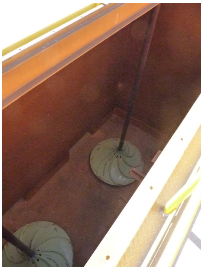
Figure 9.5. Flash mixers in a coagulation tank.
