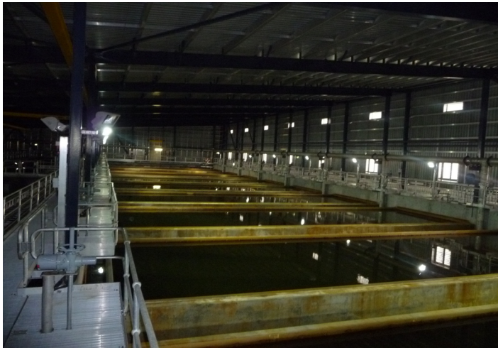
Figure 9.21. Single-stage dual media gravity filters at the Gold Coast SWRO Desalination Plant
