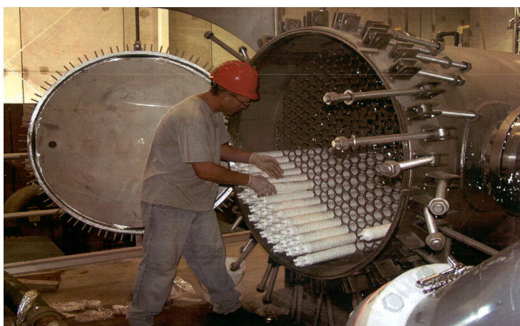
Figure 9.30. Cartridge filters installed in horizontal vessel.
