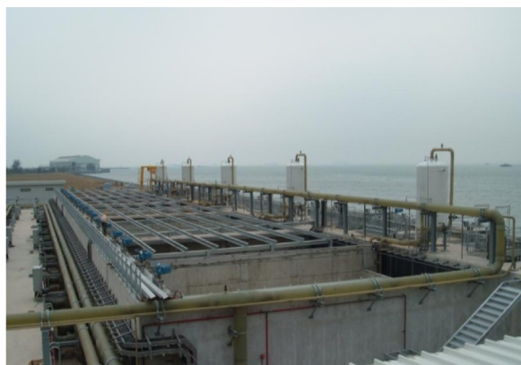
Figure 9.16. Dissolved air flotation and filtration (DAFF) installation at the Tuas, Singapore, SWRO desalination plant. Photo: PUB Singapore.
