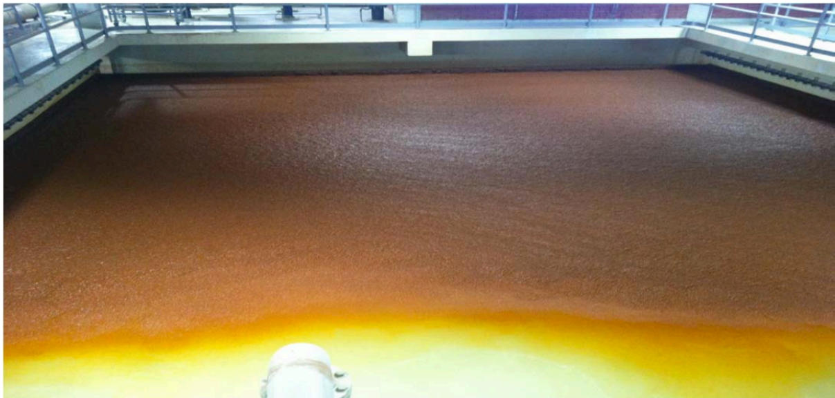
Figure 11.5.7. Floc blanket on the surface of the DAF unit.
