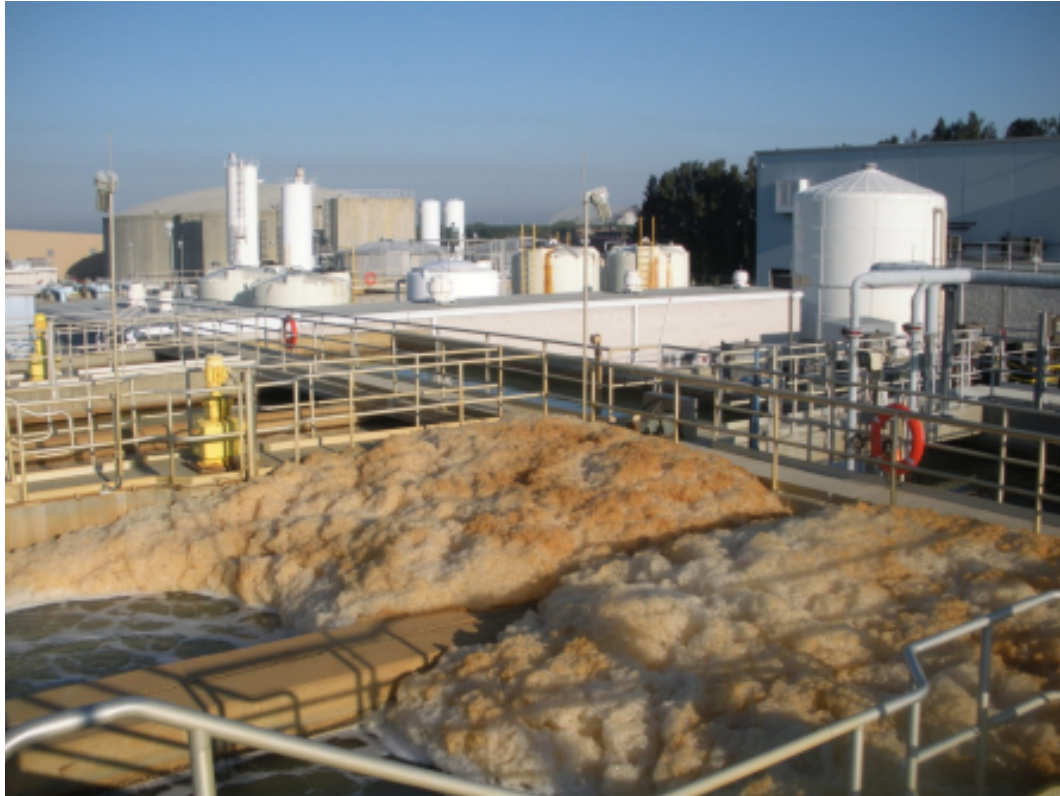
Figure 11.9.4. Foaming observed in the rapid mix basins during pretreatment at TBSDP. Source: Voutchkov (2009).
