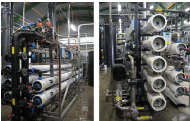
Figure 11.10.4. Demonstration plant ultrafiltration (left) and SWRO (the 5 pressure vessels on the left of the right hand image) and BWRO (the 3 pressure vessels on the right side of the skid).
