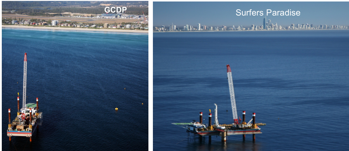
Figure 11.12.2. Self-elevating platform over intake during construction with the GCDP in the background (left) and Surfers Paradise (right).
