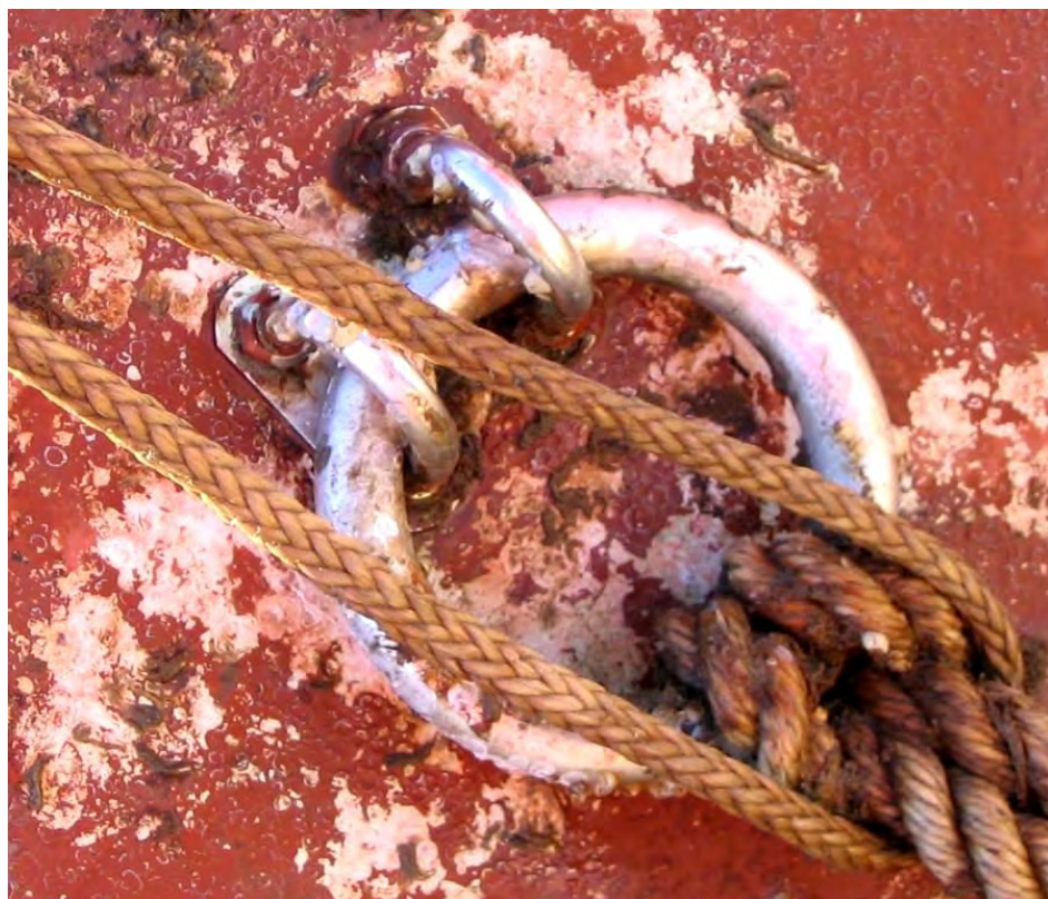
Figure 15. Intact stainless steel lift ring on the GW Bridge platform where the eye nut corroded. Most of the dark spots are paint or bio-debris
